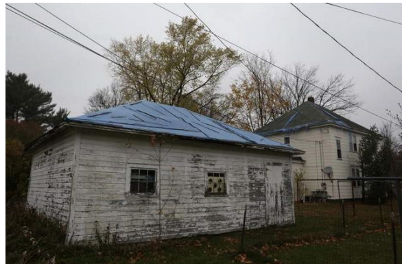
Wausau code enforcement has issued nine violations on this home since 2010.
